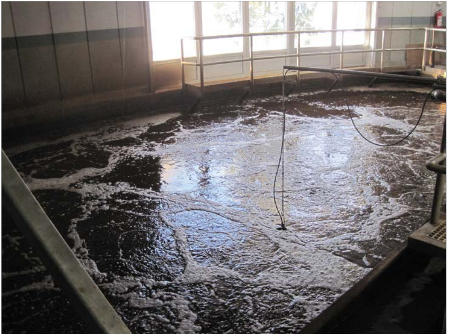
The plant's two aeration tanks are able to run in parallel or in series.
