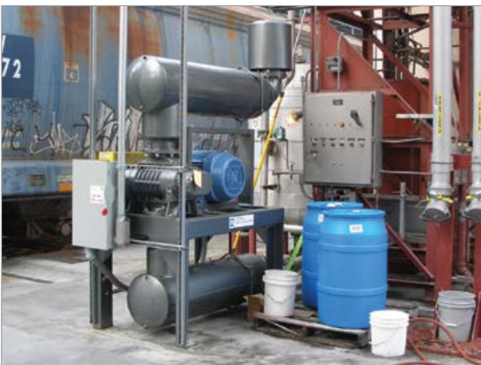
With no need to consider operating noise, this open blower package was installed outside for pneumatically conveying product into railcars.
