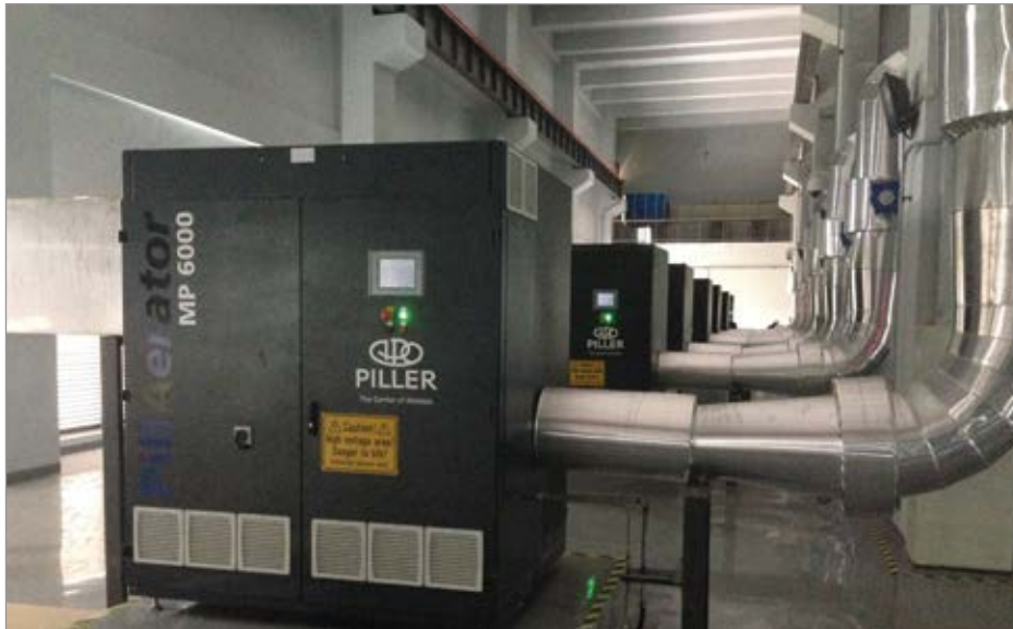
Figure 2: For yeast fermentation applications, PillAerator often installs multiple blowers to provide the proper airflow and pressure at the highest efficiency possible.
