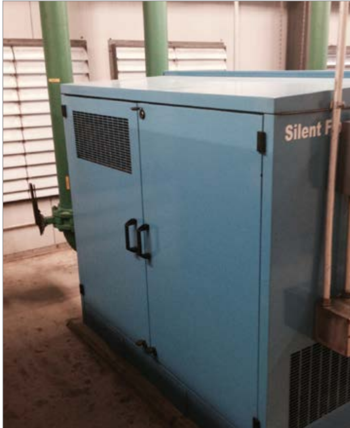
Figure 4: Existing 10-year old lobe blowers installed at the wastewater treatment plant of Hurlock, Maryland.
