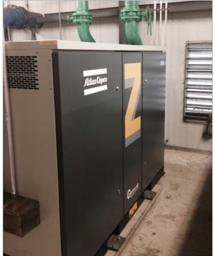
Figure 5: New Atlas Copco ZS55 blowers installed at the Town of Hurlock, Maryland wastewater treatment plant
