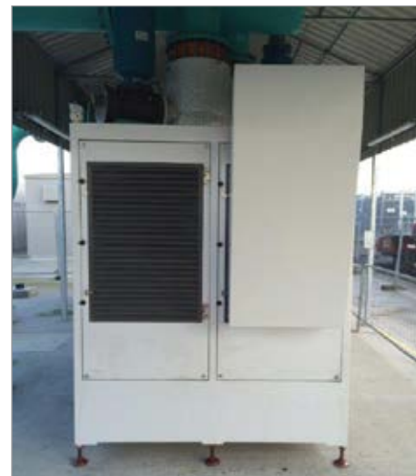
An APG-Neuros installation at Thames Water
