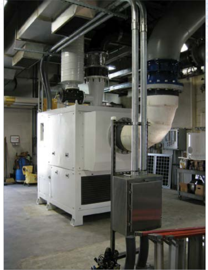
APG-Neuros turbo blower installed at the water quality control plant in South San Francisco, CA
