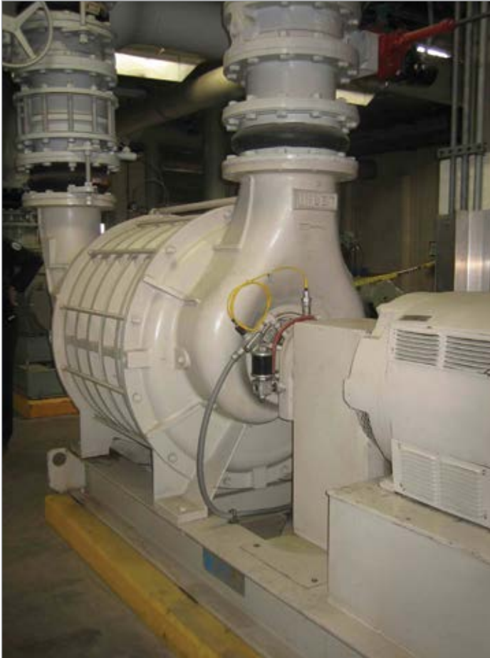
Original multi-stage blower at the San Bruno Water Quality Control Plant
