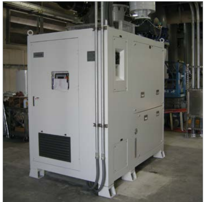
The APG-Neuros turbo blower installation received an incentive rebate worth $45,487.
