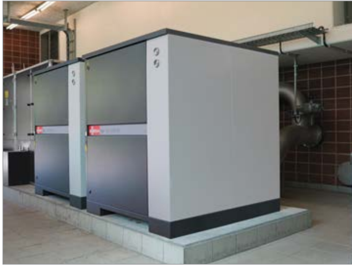
Figure 2: Two Tyr rotary lobe blowers, with an output of a volume flow of 2,600 cubic meters per hour each, are in operation on each aeration channel.
