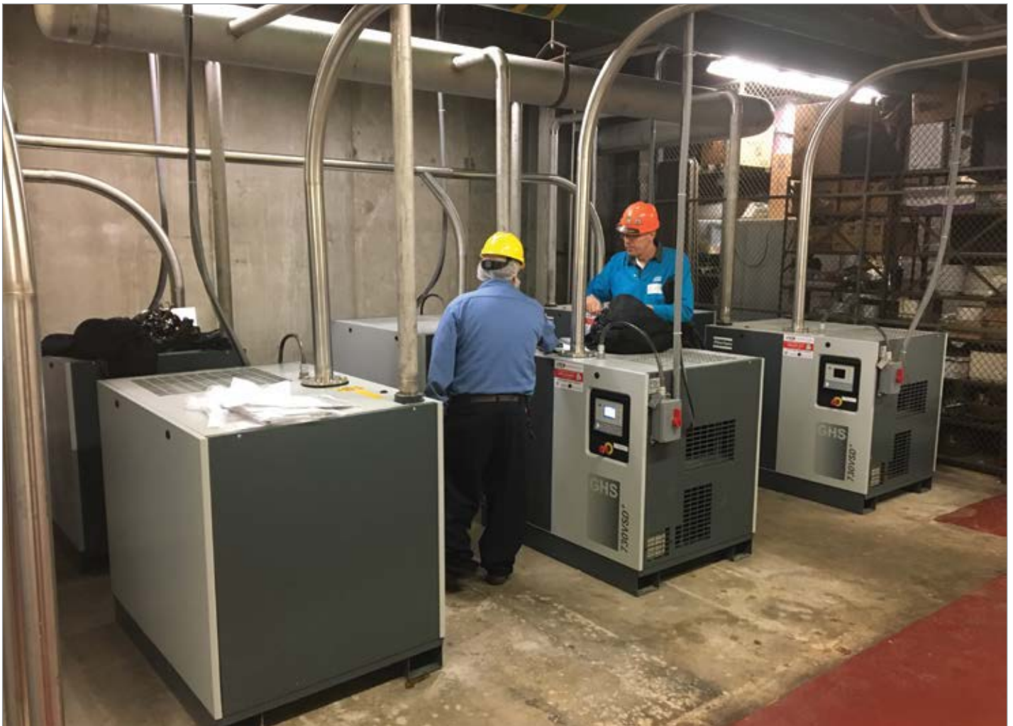
The header is recognizable, located above the vacuum pumps, more commonly seen in compressed air configurations.
