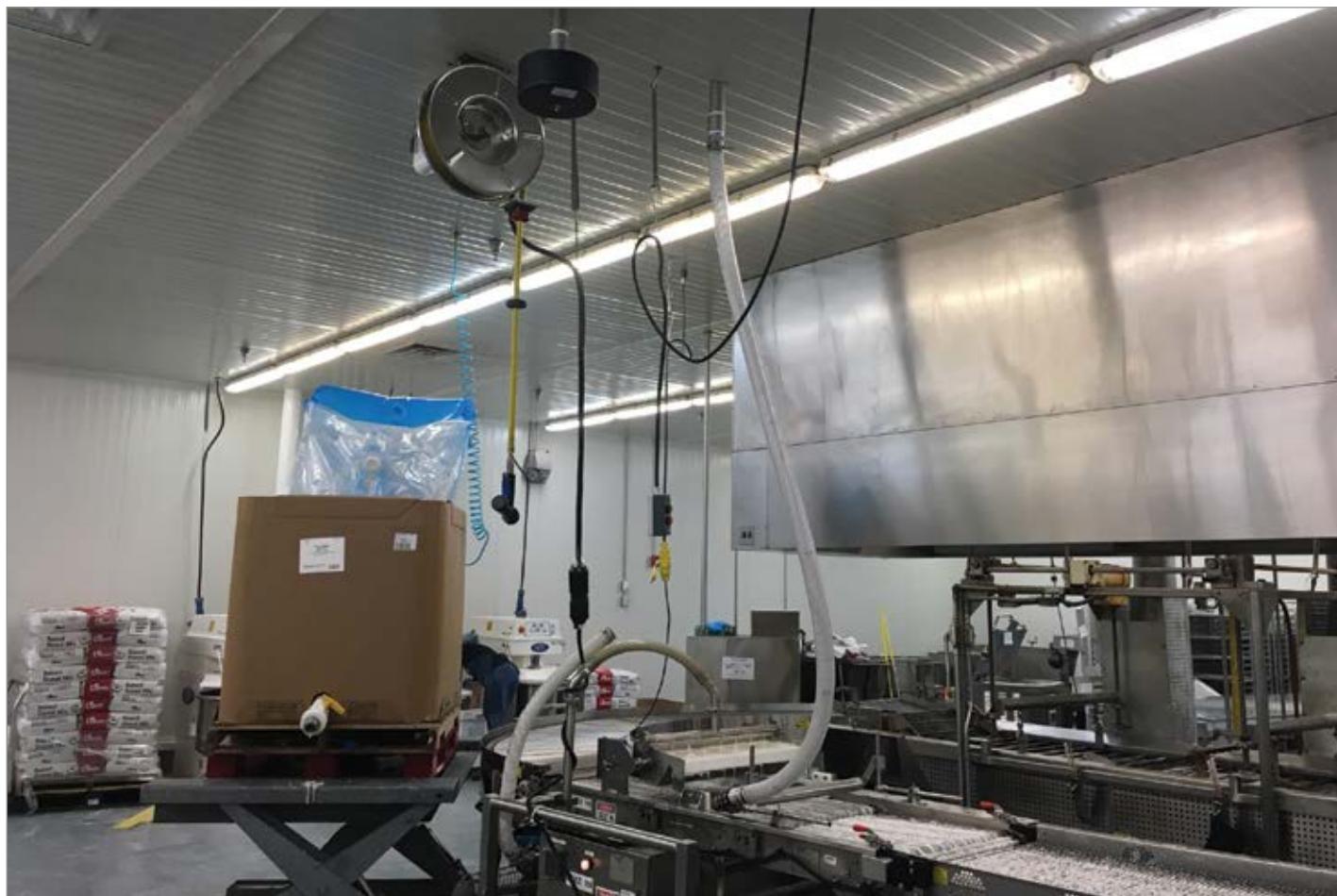
The air knife is installed and piped to the blower with a food grade hose, immediately following the application of the icing.
