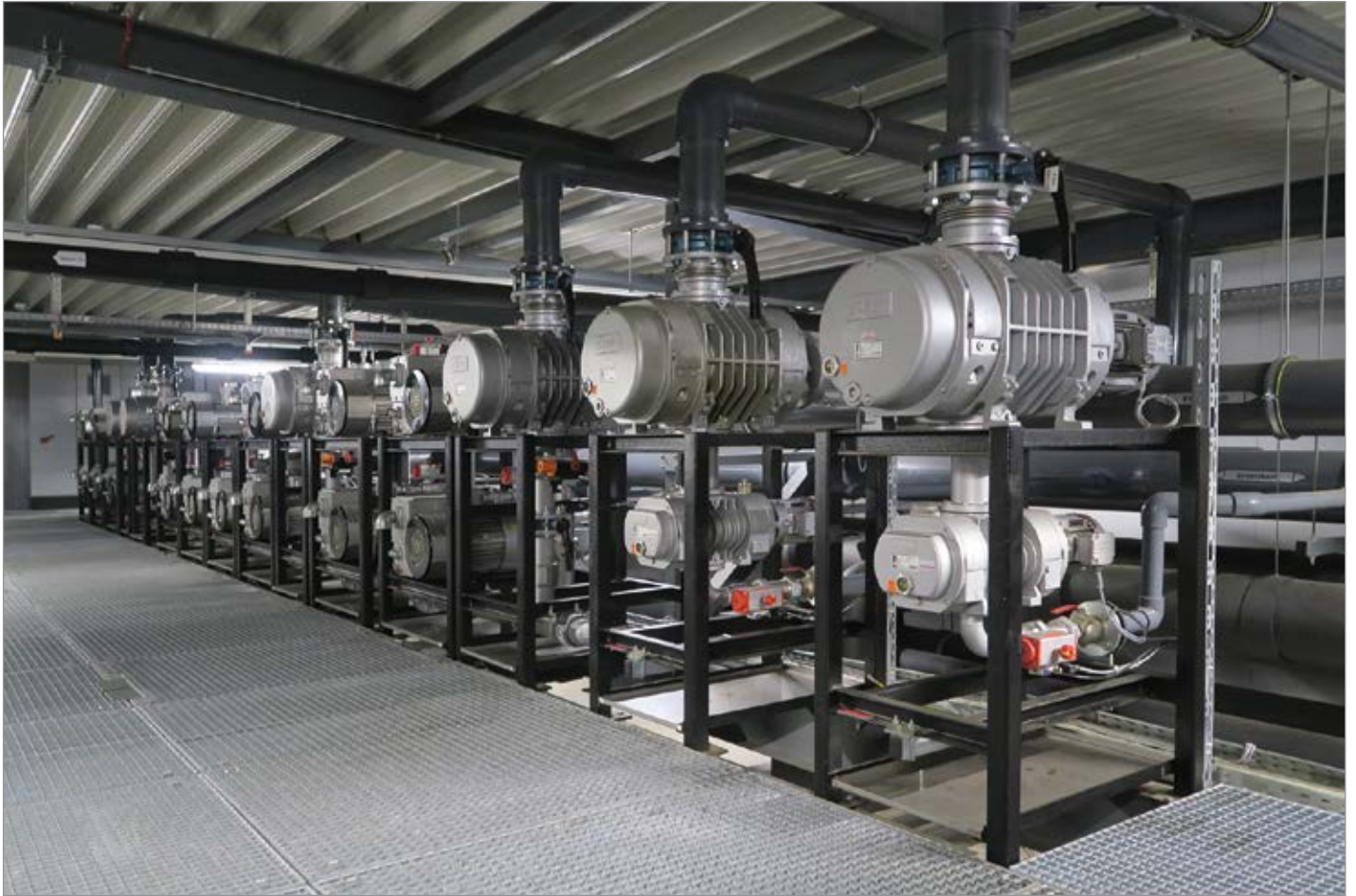
Busch centralized vacuum system for supplying vacuum to the packaging lines.
