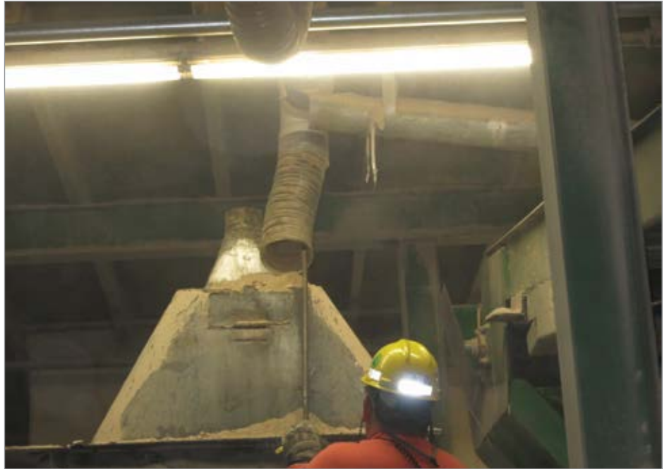
Figure 6. Typical Distribution System Leak
