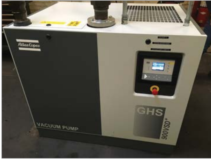
Atlas Copco GHS 900 VSD+ Vacuum Pump installed and operating at customer location.
