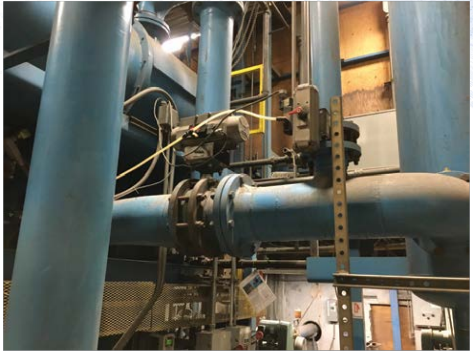
Figure 2. Typical Controlled Vacuum Demand – Furnace Pull-Down. A butterfly-valve controls flow to the furnace, to pull down a vacuum at the start of the heating cycle. It is closed when the furnace is open. Typically, there is no proportional control, just on-off.
