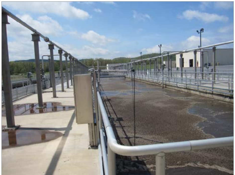
One of three NRT Reactors at the CMA Wastewater Treatment Plant.
