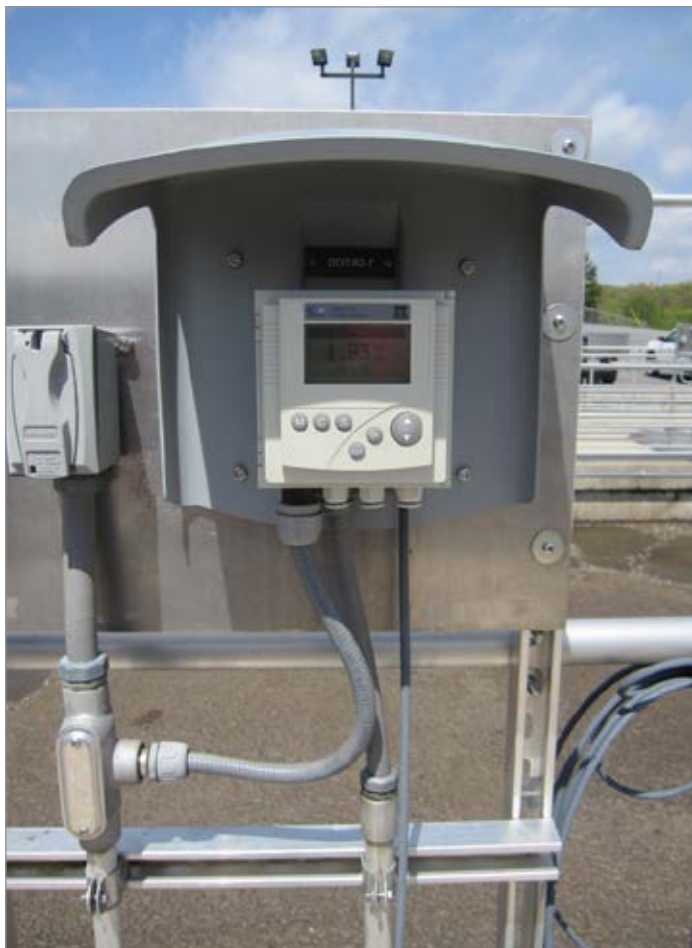
Actuator valves are used to regulate the airflow for each of the six zones within each NRT reactor at the wastewater plant.
