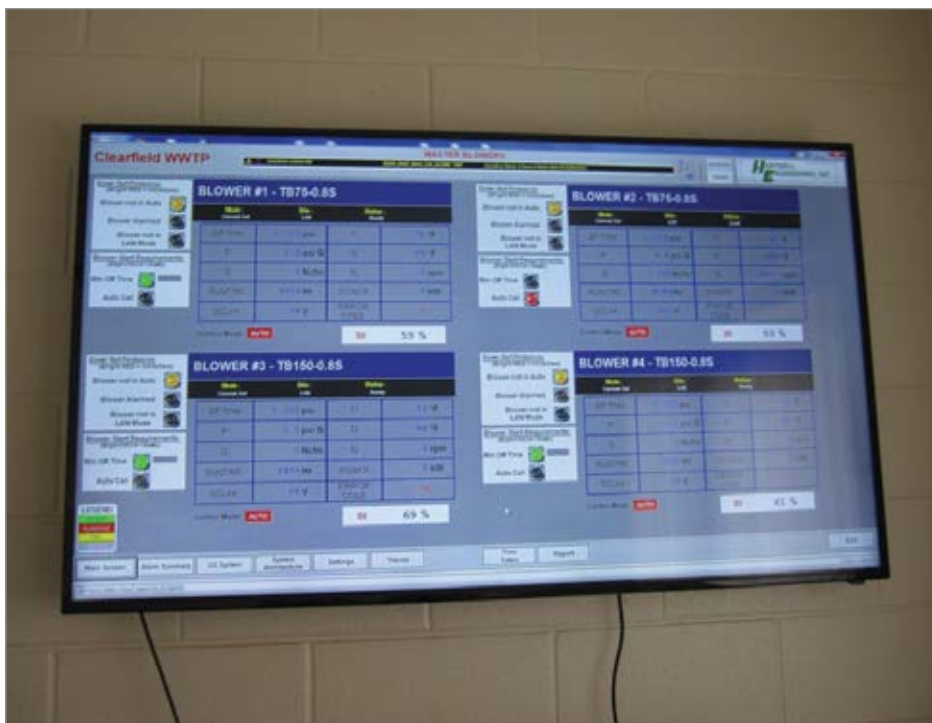
Up-to-the-minute data for blowers is visible on the treatment plant’s Supervisory Control and Data Acquisition (SCADA) system shown here. In addition, the turbo blower building and the building housing the hybrid blowers and PD blowers are each equipped with a master control panel for easy monitoring and independent control of each system.
