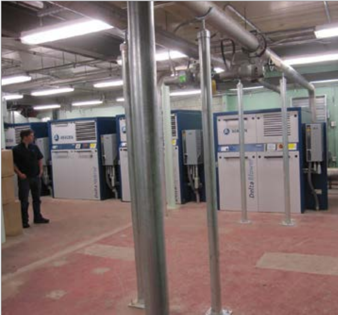
Hybrid and PD blowers are housed together in a newly constructed blower room.
