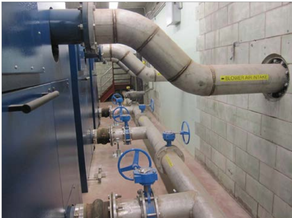
The PD blowers at the plant compress inlet air to 5.25 psi and route it through the main header (bottom) to SH tanks and the recycling tank.
