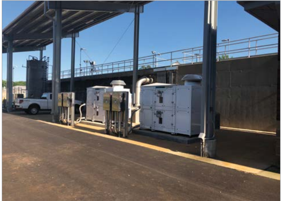
By upgrading its aerobic digesters with high-speed, integrally geared blowers, Madison Utilities’ wastewater treatment plant saves tens of thousands of dollars per year in energy costs – and gains flexibility in meeting future water treatment needs.
