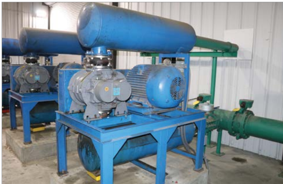
Shown are the main blowers used at the Rocky Branch Wastewater Treatment Plant in Kansas City, Missouri.
