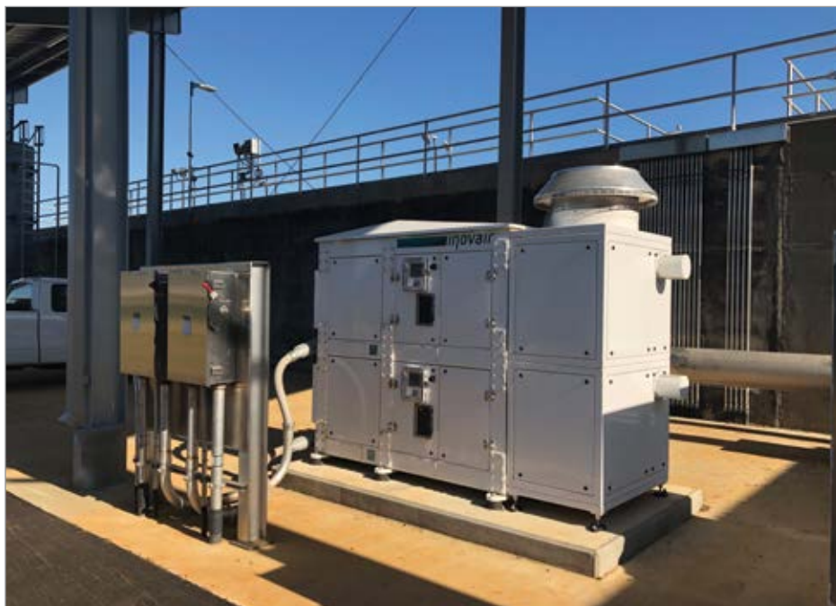
Shown is a high-speed, integrally-gearred, VFD centrifugal blower at Madison Utilities' wastewater treatment plant.
