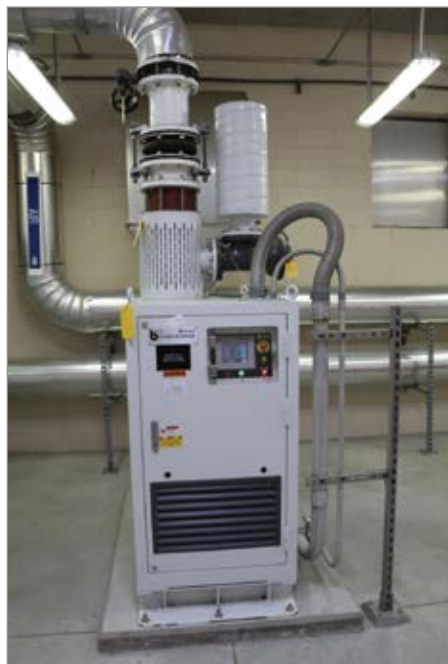
A turbo blower in use at the Fishing River Wastewater Treatment Plant in Kansas City, Missouri.
