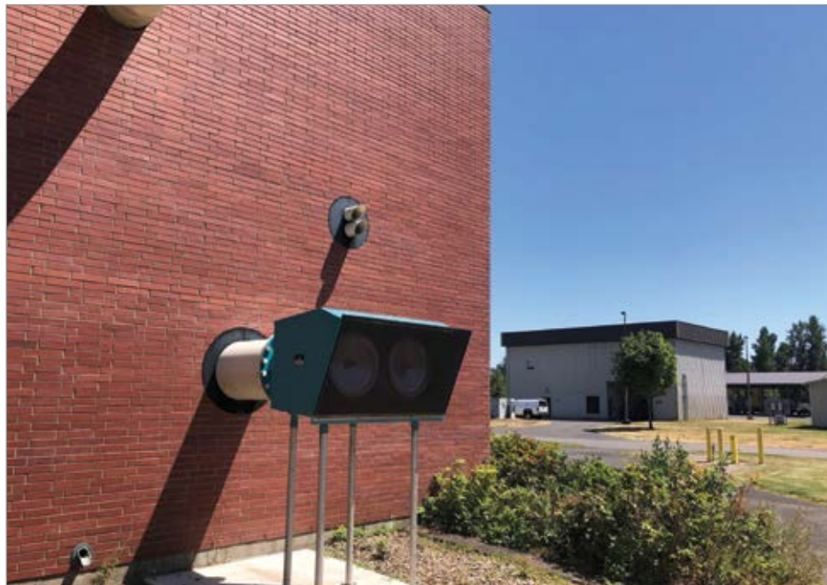
The City of Eugene installed an Endustra outlet manifold intake filter silencer at its wastewater treatment plant.
