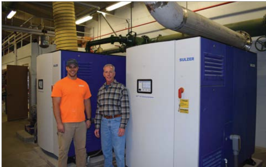
Shown from left to right are Logan Wray and Joe Fuqua of the Upper Fraser Valley Wastewater Treatment Plant. (Photo courtesy of Sulzer Pump Solutions, Inc.)
