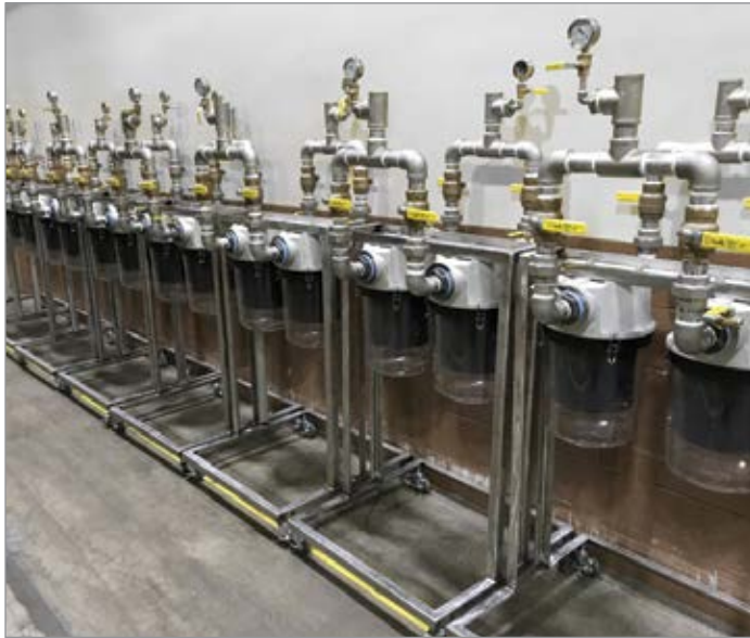
This bank of Solberg ST style particulate filters protects vacuum pumps from dust and flakes produced during a consumer goods packaging process
