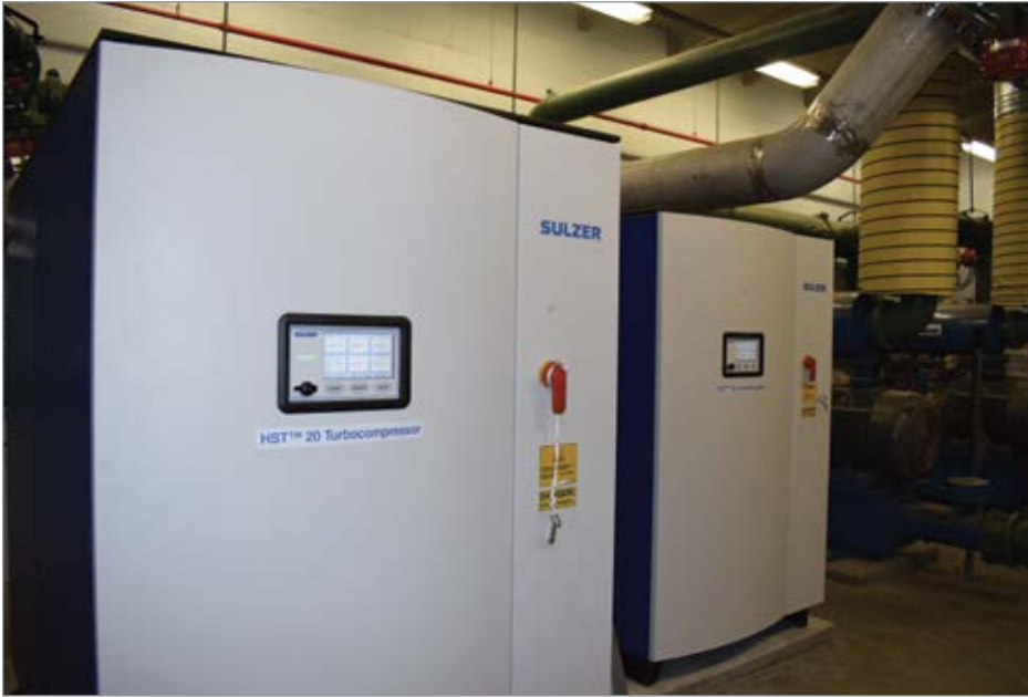
Sulzer HST turbocompressors provide aeration to the Fraser wastewater treatment plant's aeration basins and digester tanks. (Photo courtesy of Sulzer Pump Solutions, Inc.)
