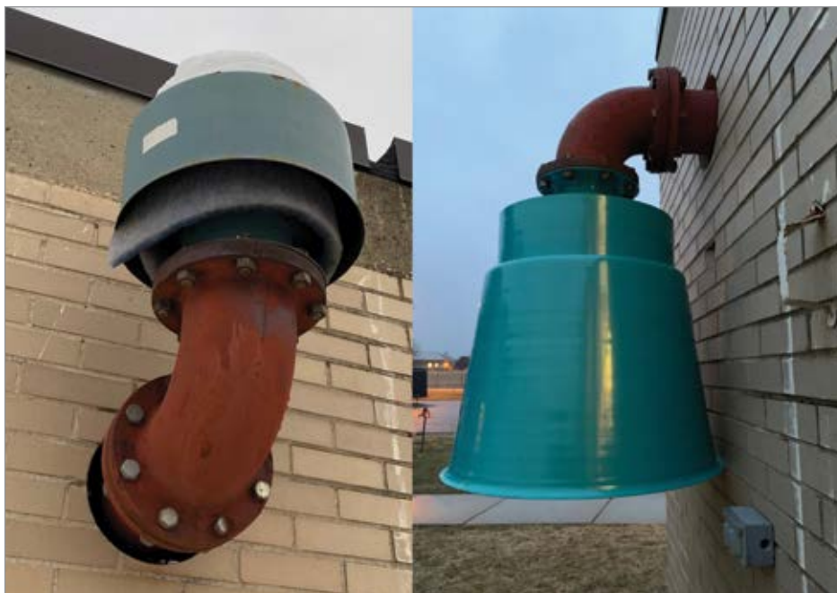
The St. Charles wastewater treatment plant reduced its energy costs and addressed safety and noise concerns by replacing the original blower inlet filter (left) for its multistage blowers with a new inlet filter silencer (right).
