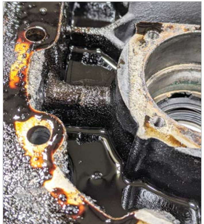
All oils wear out, creating the potential for sludge buildup.
