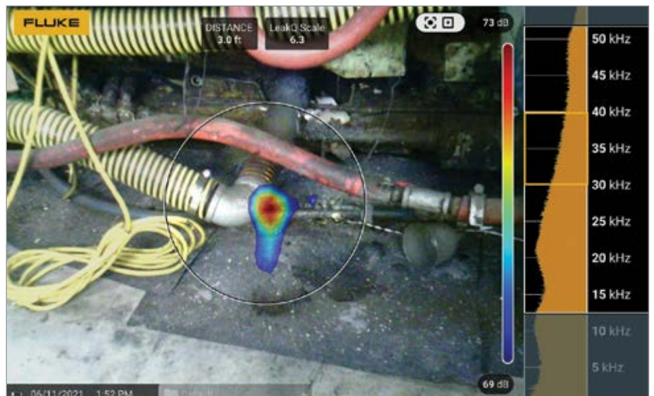
Profile of a Fluke acoustic imager showing large vacuum leak on production machine. The compression connector was only hand tight in this case, but the vacuum force held it onto the machine.
