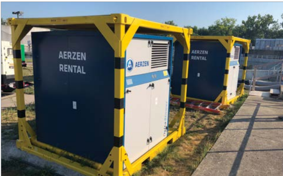
Temporary aeration blowers installed at a wastewater treatment plant.
