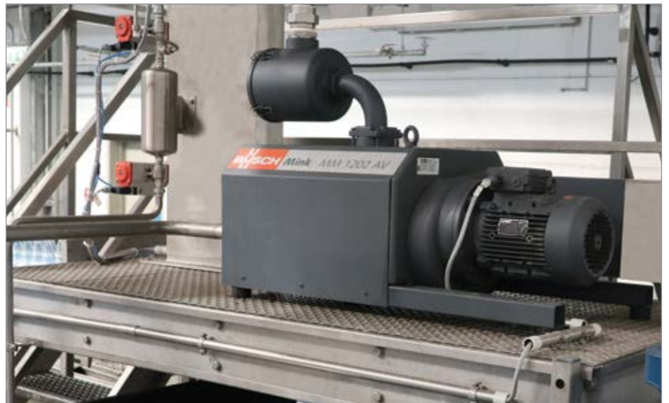
Figure 2. MINK claw vacuum pump for degassing the well water in the degassing tank.
