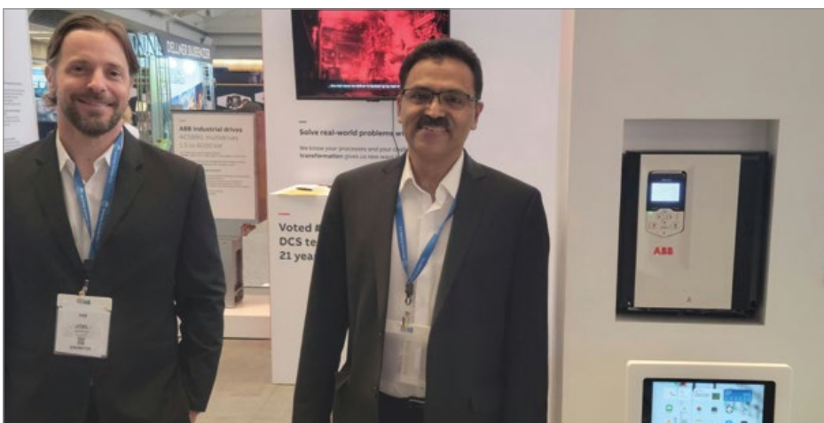
Joel Hatfield and Siraj Boudighar (left to right) next to ABB's control system.
