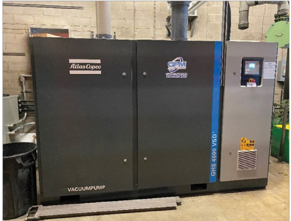
Figure 4: The new VSD pump is more efficient, produces less heat, and is much quieter than the old pumps.
