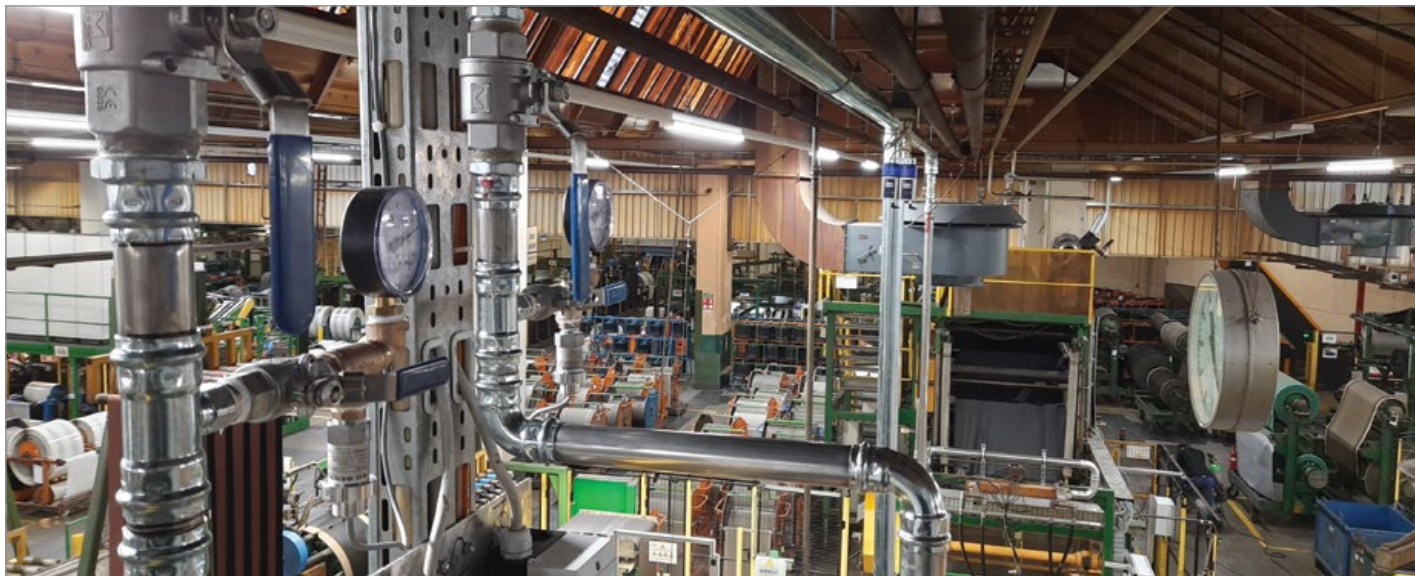
Piping system for the vacuum supply of the textile-cutting machines at Continental Reifen Deutschland GmbH. Photo: Busch Vacuum Solutions
