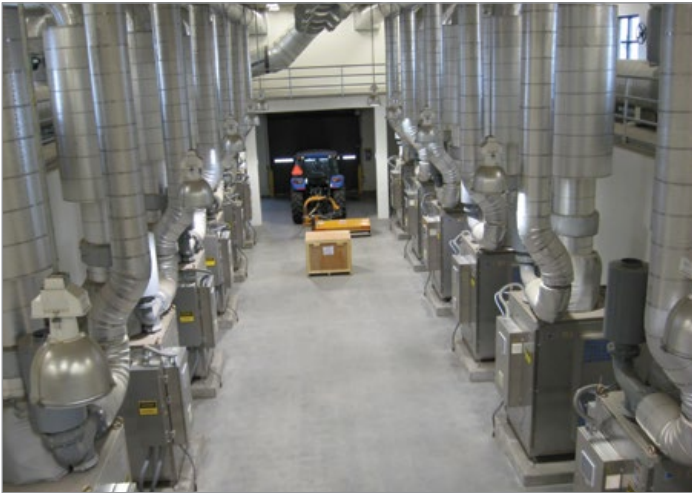
Figure 1: Example Blower Room Layout with Housekeeping Slabs and Generous Spacing for Service Access
