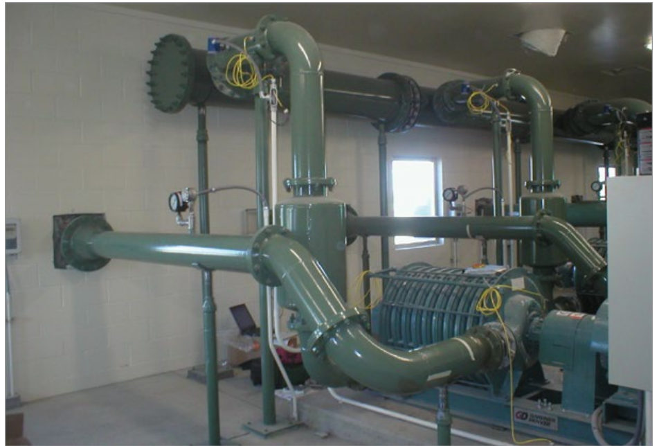
Figure 2: Example Blower Room Layout with 45° Connection to Carbon Steel Discharge Header (Upper Pipe)
