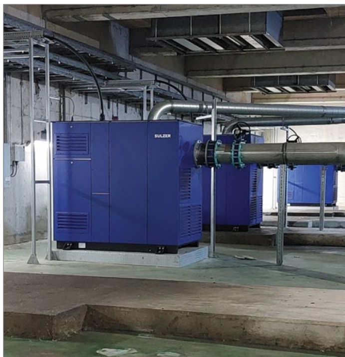
Six HST 20 turbocompressors from Sulzer were chosen to replace eight units at Derby Sewage Treatment Works to reduce the risk of downtime.
