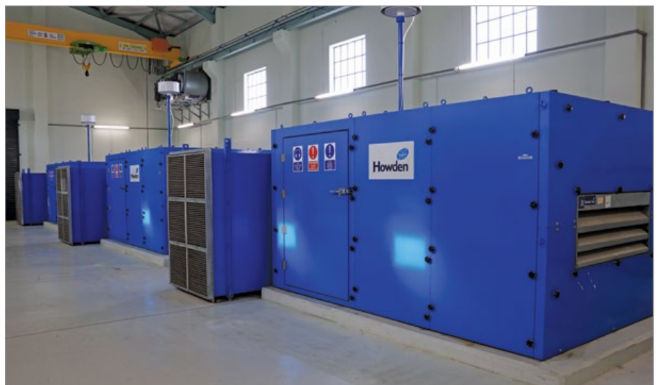
Howden supplies energy efficient aeration solution to Athlone Wastewater Treatment Works.
