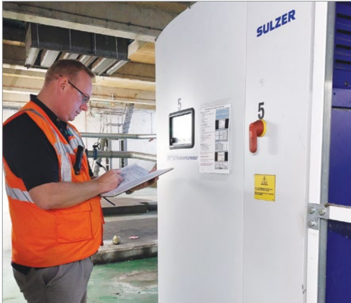
Severn Trent's Health and Safety team confirmed that historical noise restrictions could be removed, so operatives working in the blower house basement no longer needed to wear ear protection.
